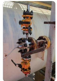
Flushing Ring in HF Process
